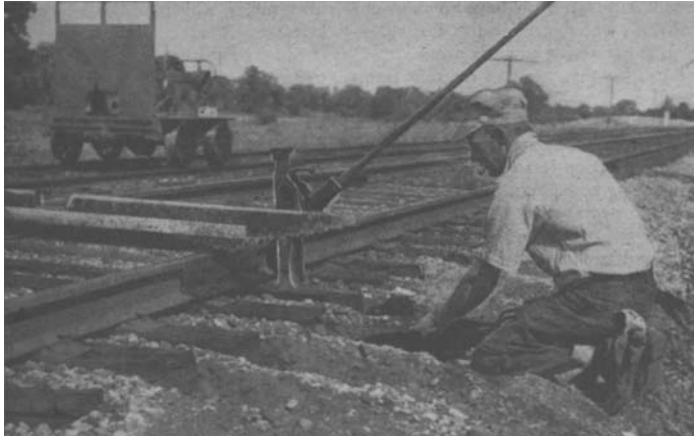
"Bob White [the article's author] is shown here, 'shooting' modern ties on the Grand Trunk Western. Ballast is first removed from the ends of the ties. The track is then jacked up and fine stone slipped under it atop a thin blade. The latter is then withdrawn quickly, leaving ballast in place"
