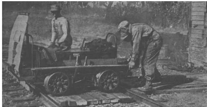
"Illinois Central buzz-wagon being set on the rails at Seward, Illinois, by 'King Snipe' Alfred Schere and two of his men"
